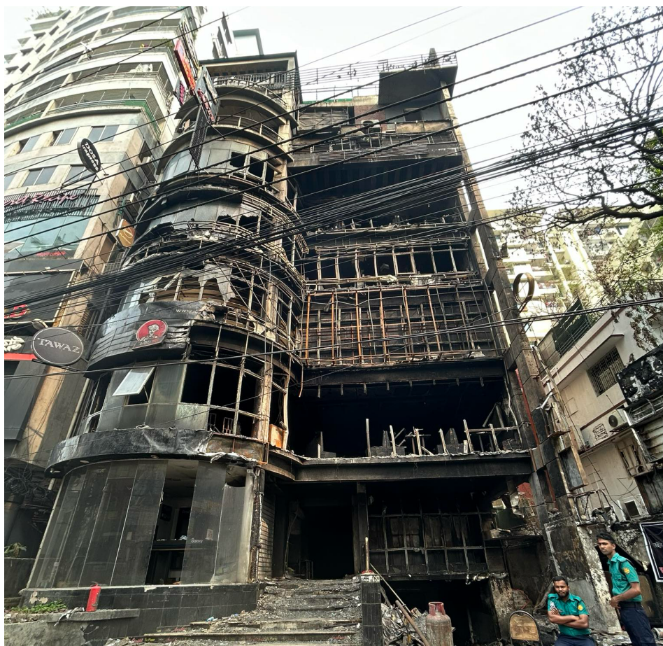
Figure 08: Damaged building and exterior glass wall
